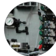
Pneumatic control systems
